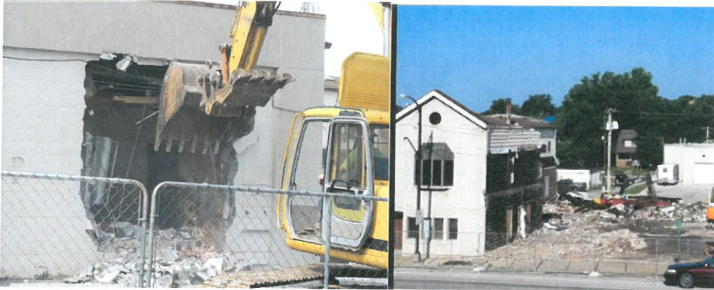
Demolition began on June 18 th and is supposed to be completed in 30 days.
