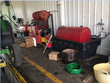
Figure 11: Clifton Facility petroleum storage indoors with secondary containment
