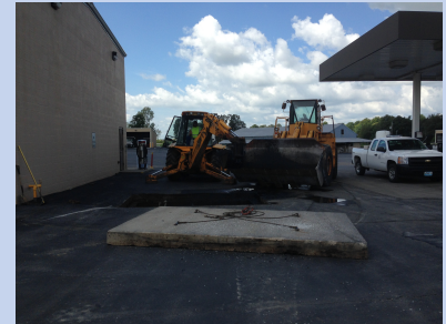
Figure 7: Vehicle wash bay separator cleaning
